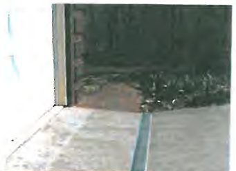
Installation of a channel drain as part of a stormwater management system prevents damage to the house and landscape from excess water.
